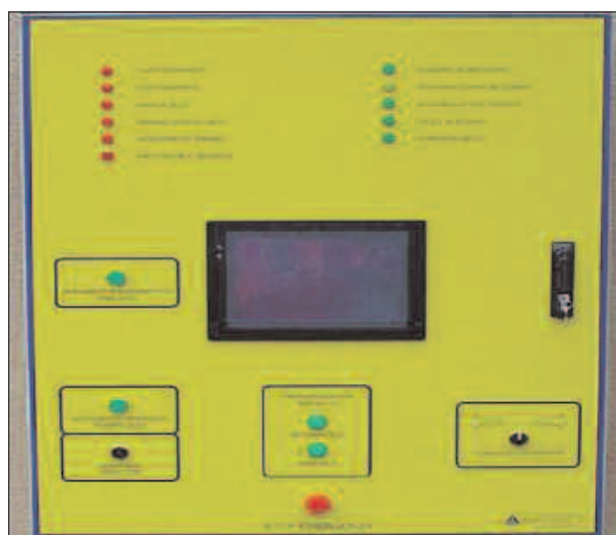
The auxiliary control panel
