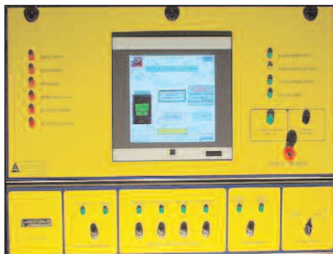
The main control panel
