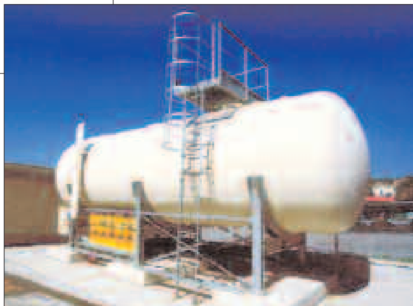
The tank for saline solutions
