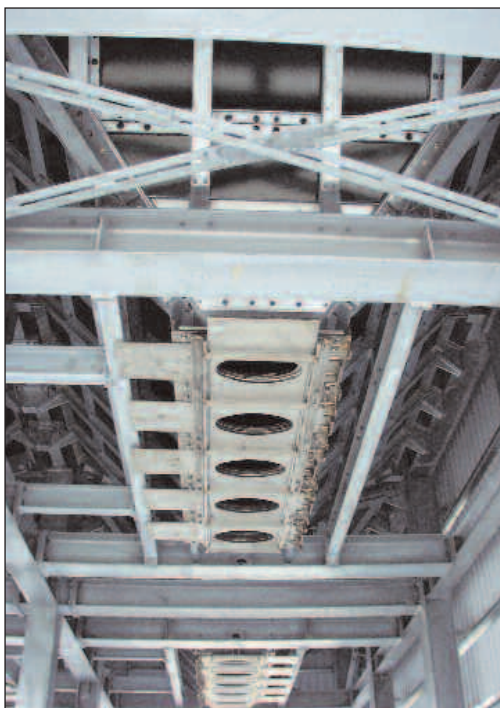
The discharge gates with five openings under the individual hoppers
